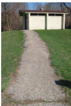
Restroom path (note condition of walkway)
