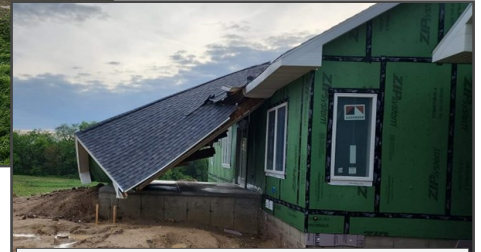
A new construction home could not sustain the 75mph winds.
